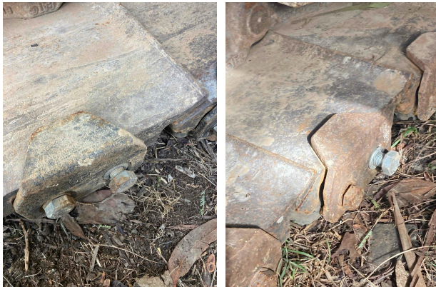
Image Comment(s): Loose mounting bolts
